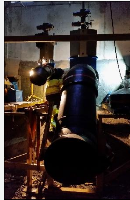
Outlet valve & pipe
