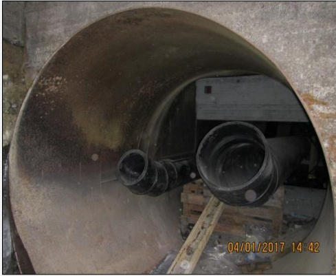
Outlet pipes (for Sluicer and Gravel Excluder)
