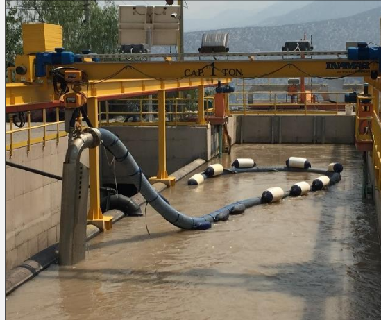
Desander with SediCon removal equipment
